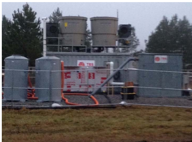
Figure 9. East Side Equipment Compound
