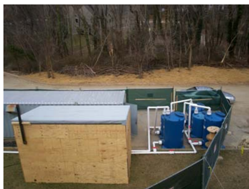
Figure 4. ERH Equipment Compound with Sound Enclosure (plywood) around Blower
