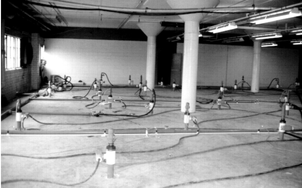
Figure 3 - Electrode/Wells Inside Building
