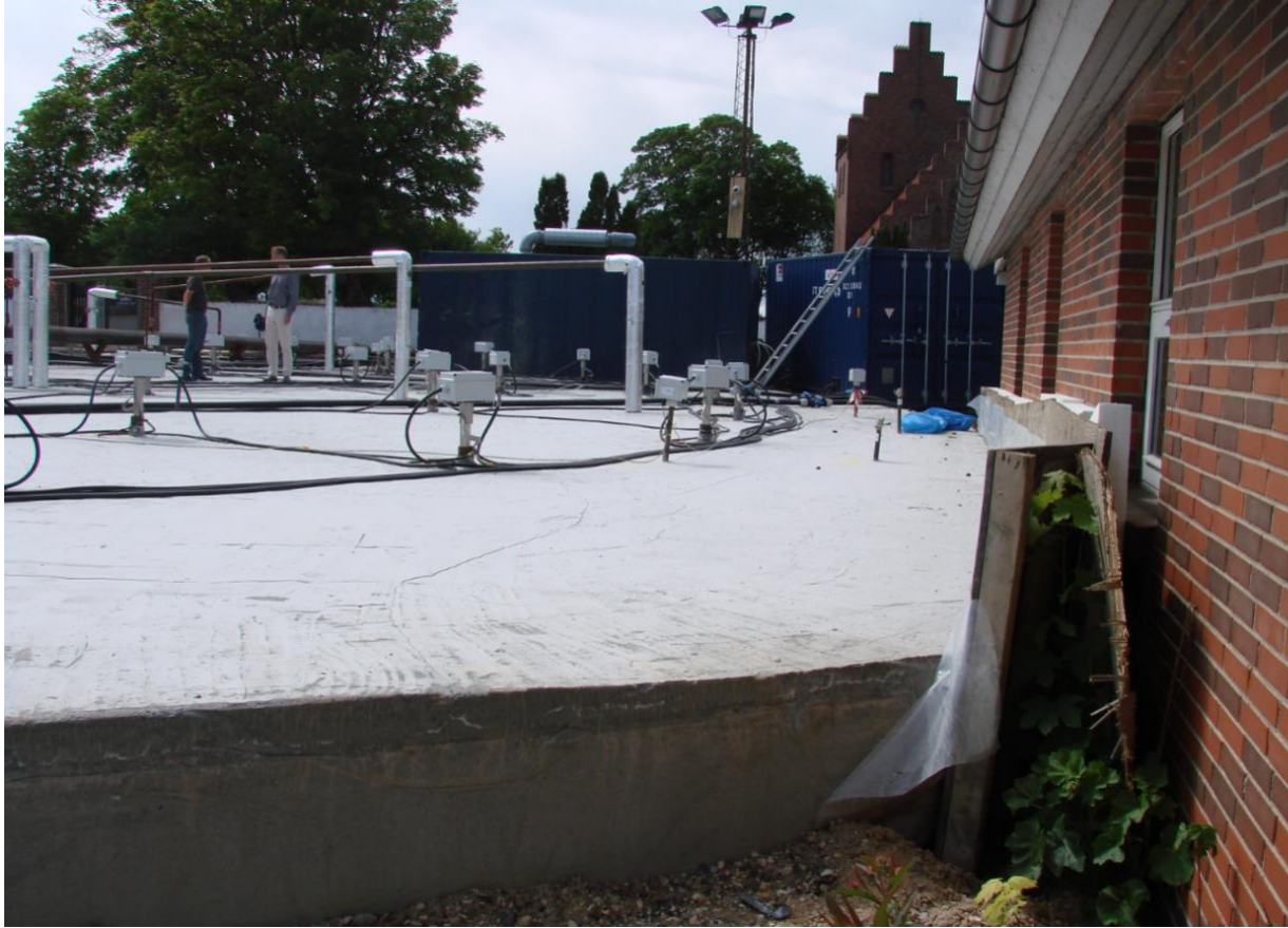
Figure 2. TCH remediation of a 9 meter deep clay layer heated to 100°C next to a building – no subsidence observed (Reerslev, Denmark; Kruger and TerraTherm, unpublished).
