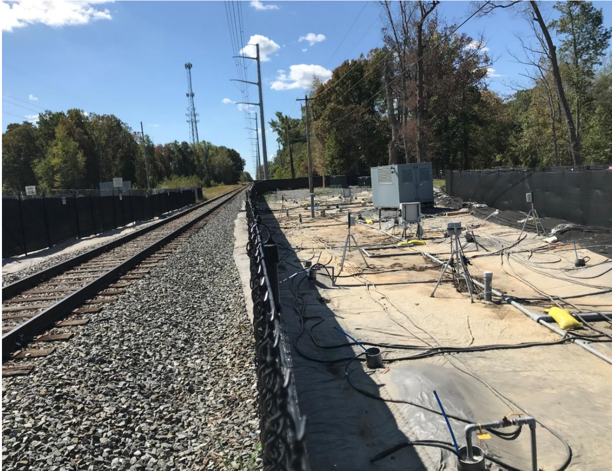
Figure 3. ERH operation under an active railroad – electrodes were placed under the railroad, and the subsurface was heated to boiling temperatures without any adverse impacts (Brandywine, MD; TRS Group, unpublished).
