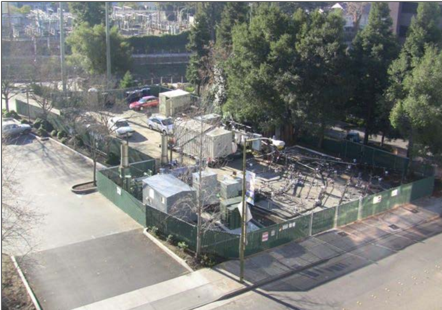
ERH treatment area and equipment compound
