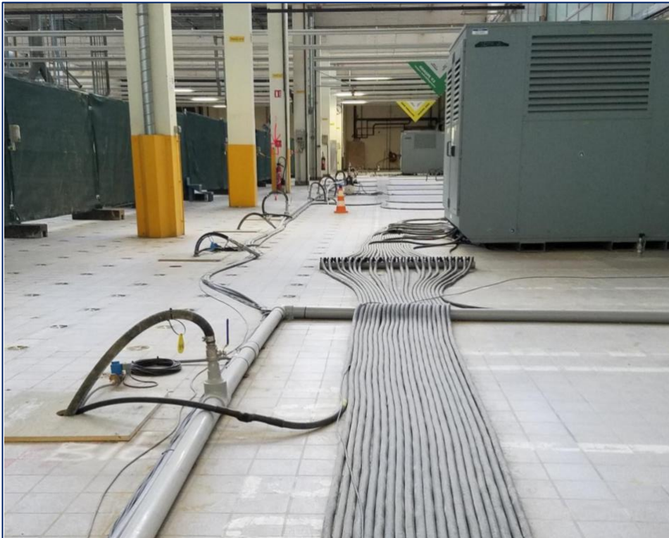
Basement Area Electrodes
