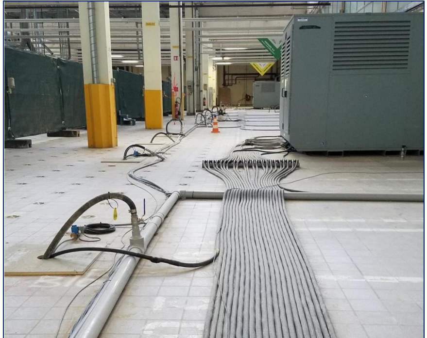
Basement Area Electrodes
