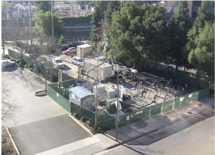
ERH Treatment Area and Equipment Compound
